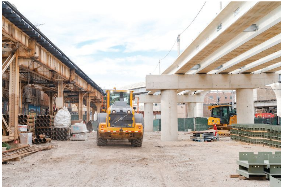
Precast, prestressed concrete beams on the new structure adjacent to the existing, deteriorating steel structure. Photo: Walsh-Fluor Design-Build Team.
