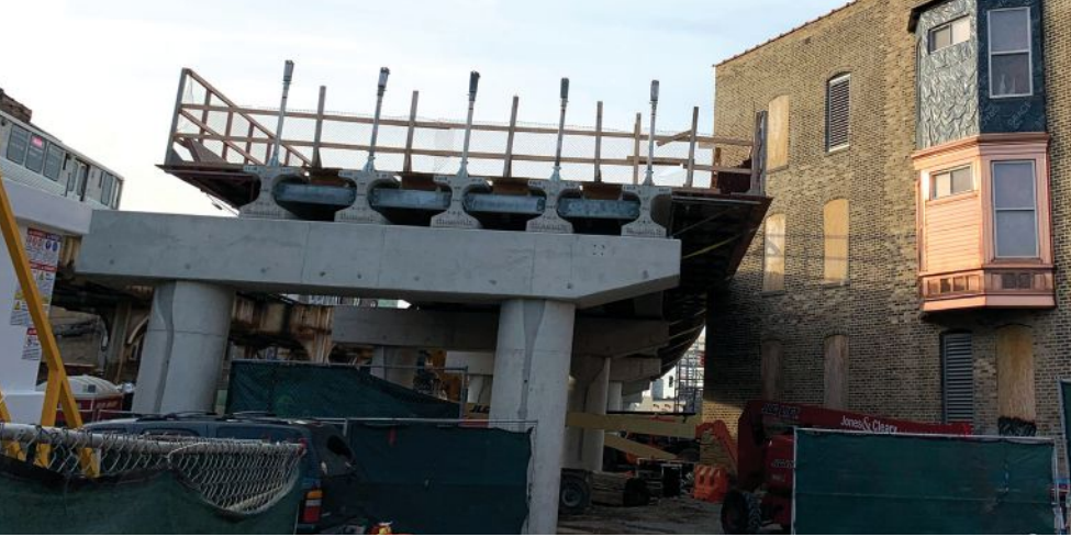
Precast, prestressed concrete beams with deck formwork are adjacent to the historic Vautravers Building, which was relocated approximately 30 ft to eliminate a curve in the existing rail alignment. Photo: Stantec.
